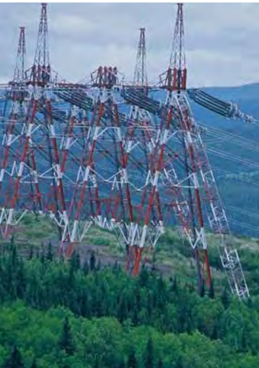
Hydropower transmission lines are one of the lesser-known and less-discussed environmental impacts of hydropower.
