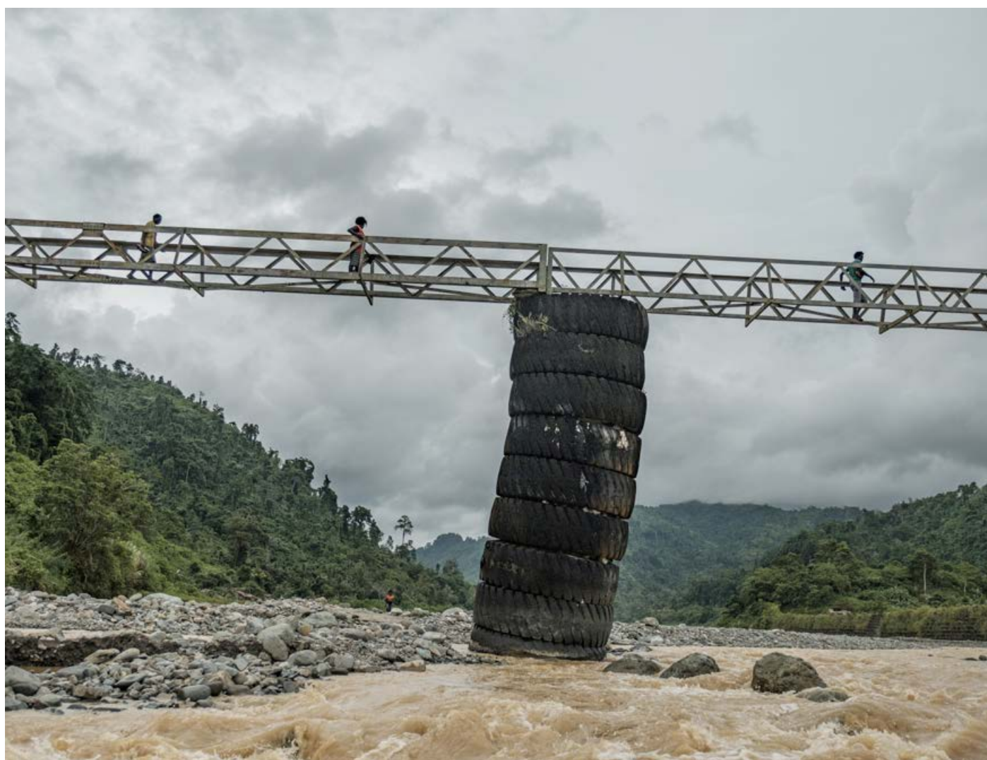
Collapsing tyre bridge, Middle Tailings.
