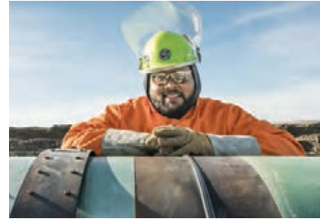
▲ In August 2017, we broke ground in Canada on our Line 3 Replacement Program—the largest project in Enbridge's history—which will enhance the safety, operational reliability and throughput of the Mainline System.
