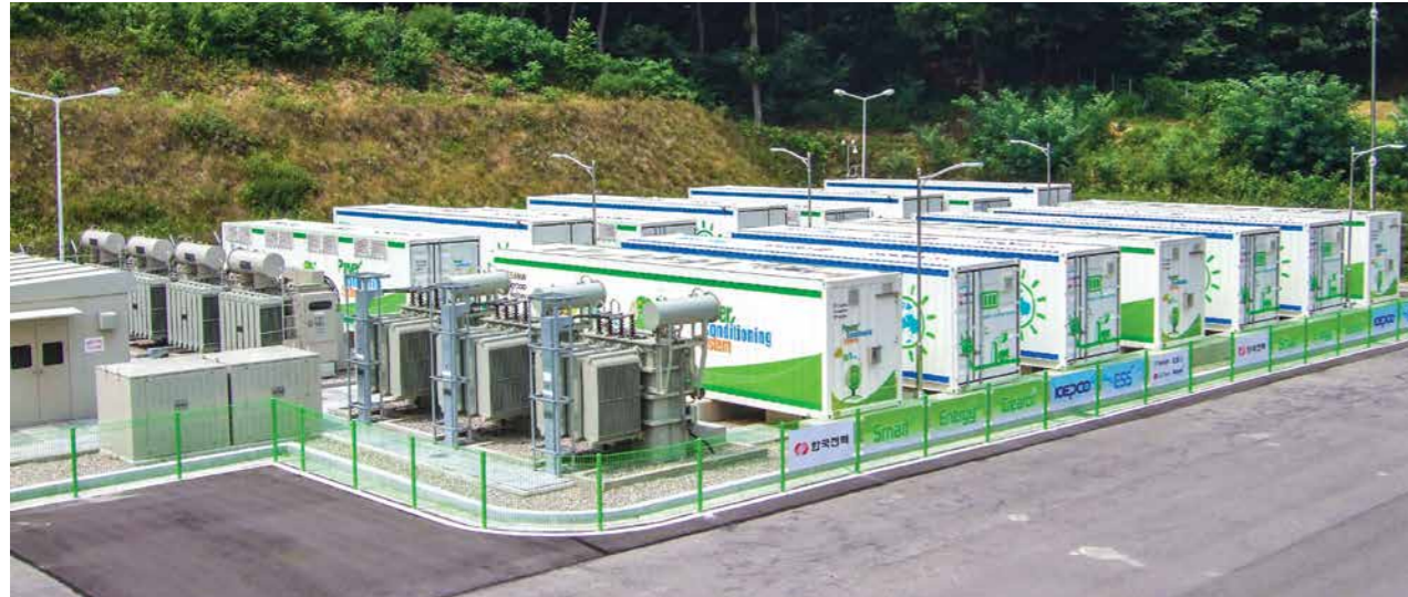
Frequency-regulating ESS at Seo-Anseong substation
