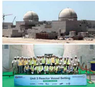
[Top] UAE nuclear reactor construction site / [Bottom] Groundbreaking ceremony for #3 nuclear reactor in Barakah, UAE
