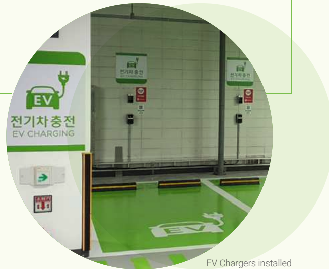
EV Chargers installed at the KDB HQ
