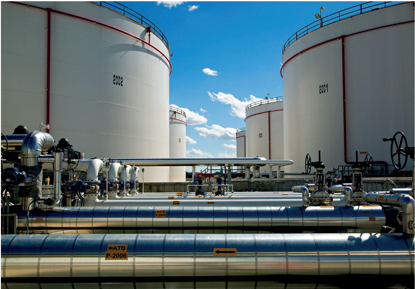
Fuel storage at Corpus Christi terminal, Texas, US.
