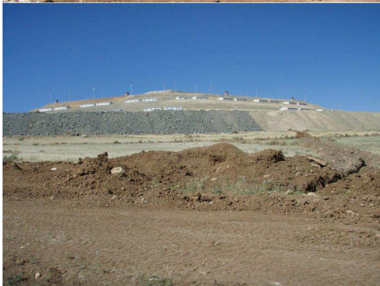
Photo 15: Camp security Military camp at entrance to construction site, carried out with massive earth movement. May 2008
