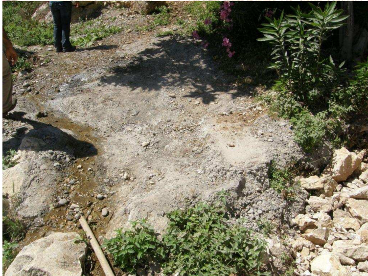
Photo 11: Unnecessary concreting Surfaces covered with concrete without any specific purpose. This as well is an unnecessary impact. May 2008
