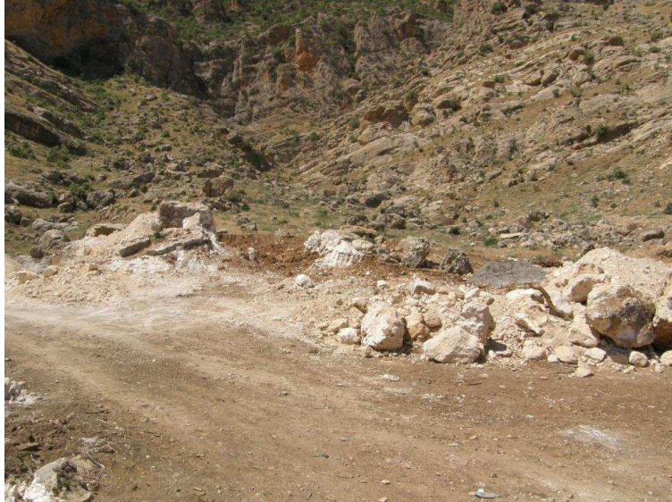
Photo 14: Road to water intake The disturbed surface is much larger than what would have been required. This can be prevented by clearly marking the area to be used before work starts. May 2008
