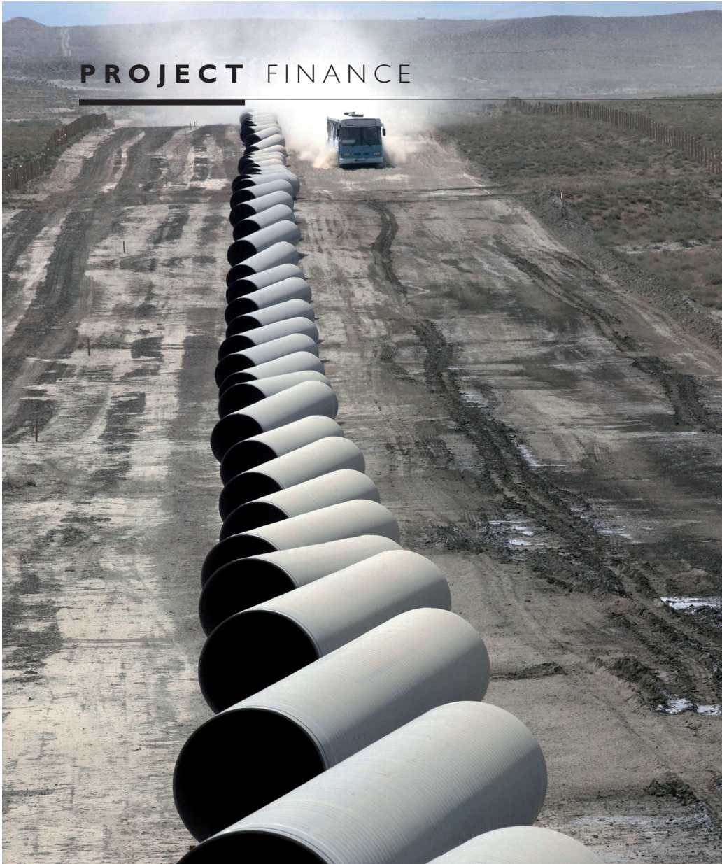
Building the BTC pipeline – but can banks build in better environmental risk management?
