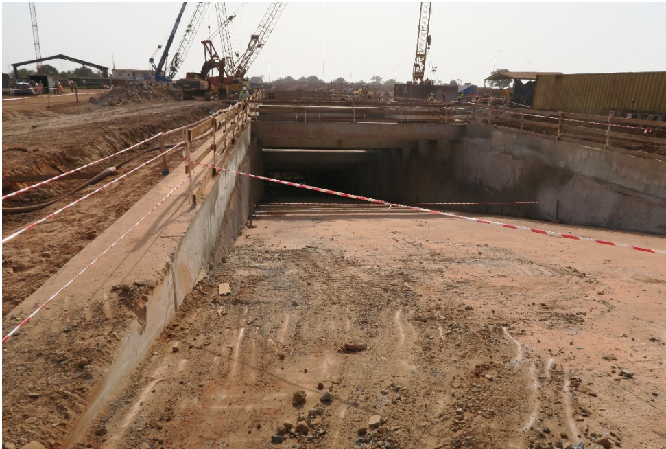
Photo 5. Exit ramp from the primary crusher pit to secondary crusher
