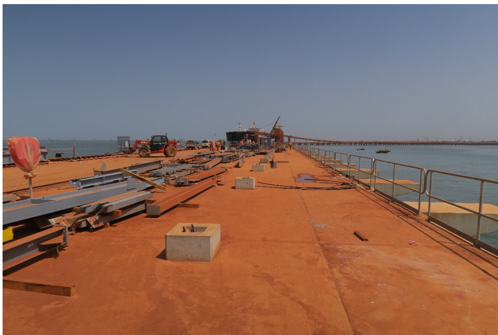
Photo 14. Extended jetty with original jetty in the background – awaiting construction of conveyor
