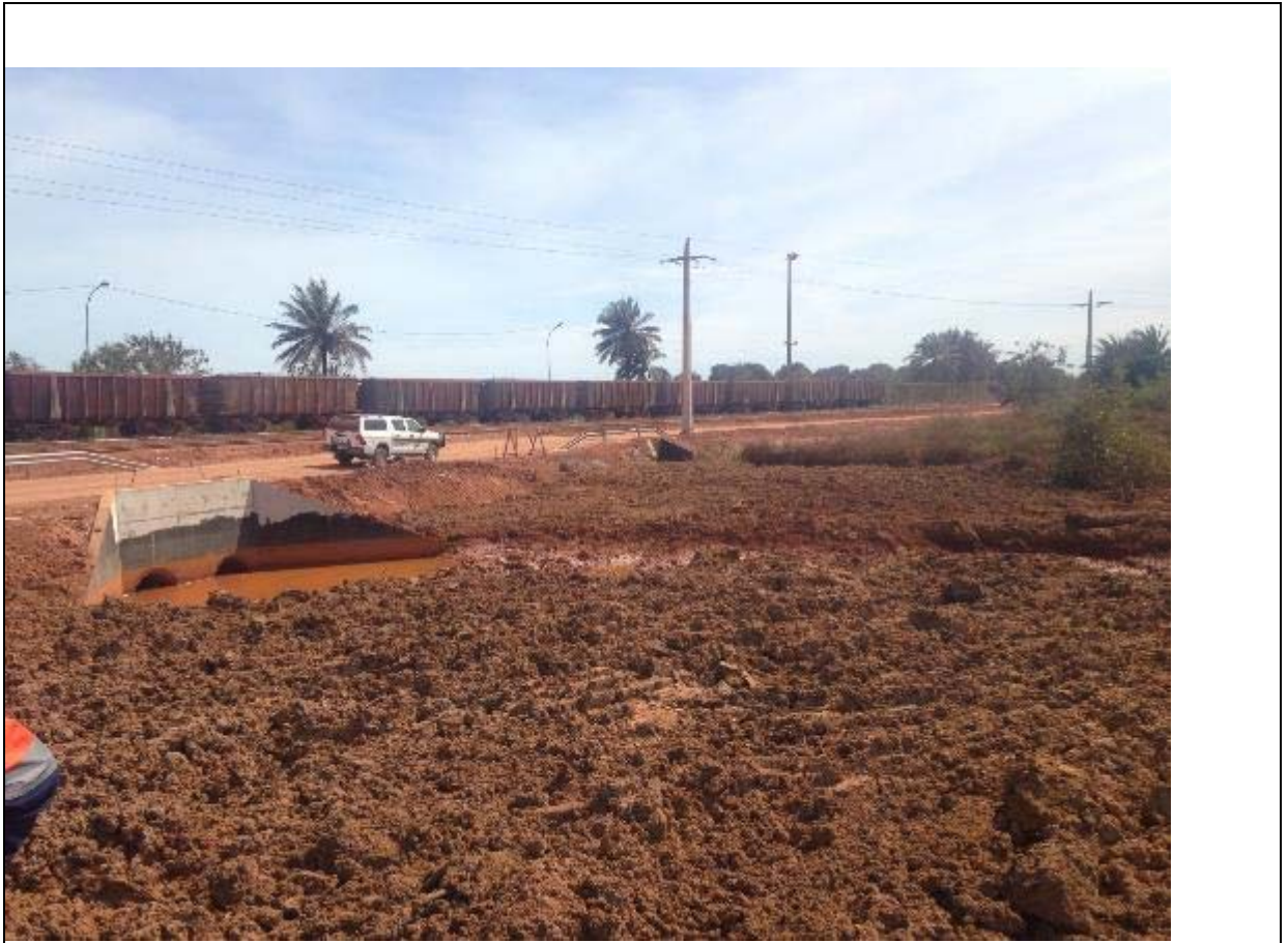
Figure 25: Area of Damaged Mangrove
