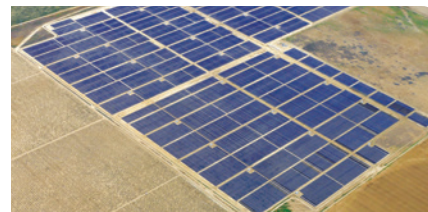
This Solar Flow-Through Fund 600 kw DC site, which is located in the Greater Toronto area, was serviced by Panasonic and PNC Canada. For the next 20 years, this project will produce green electricity for Ontario's electrical grid.
