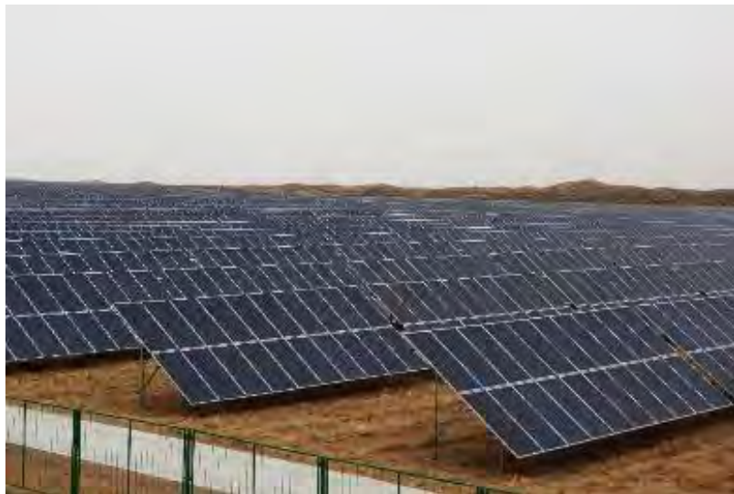
Gansu Branch contributes to the development of local photovoltaic and wind power companies (Photo by Wu Peng)
