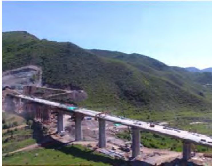
ABC supports the construction of Qingyanggou bridge in the Beijing-Zhangjiakou high-speed railway
