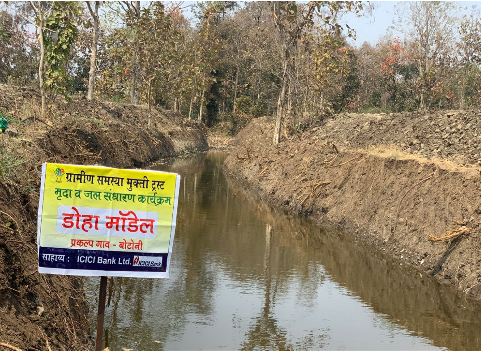
Canal deepening and widening work under the Watershed Development Project in Yavatmal district, Maharashtra
