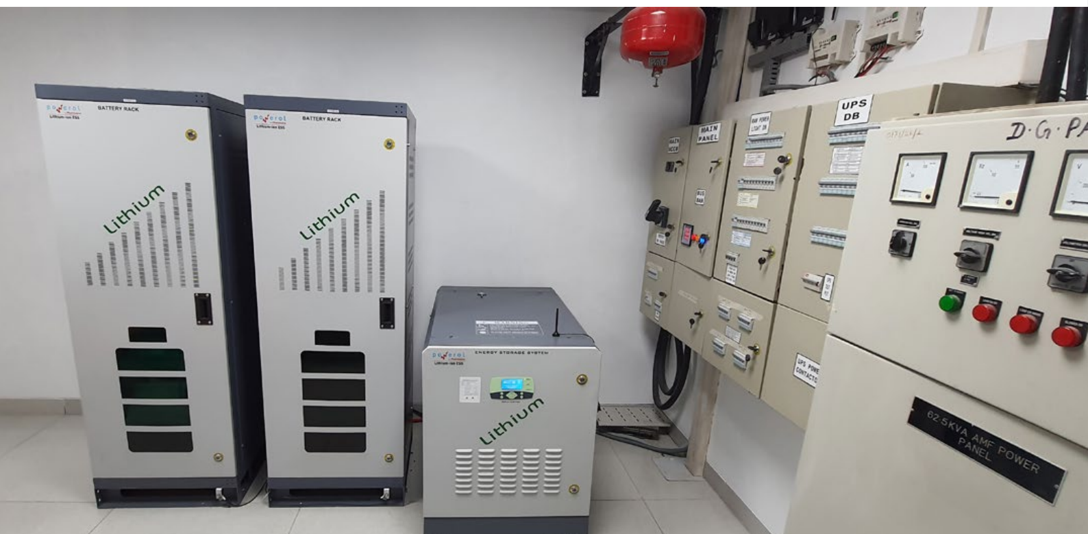
10 Kva inverter and Lithium-ion battery installed at an ICICI Bank branch in New Delhi
