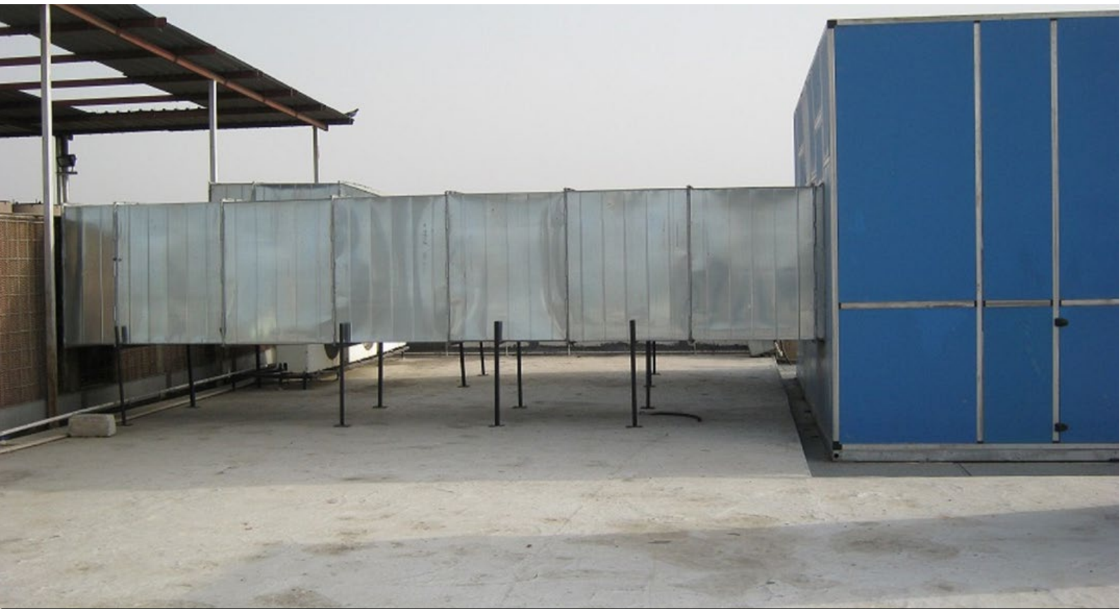
Unit for waste air utilisation under the IDEC project at ICICI Bank’s office in Jaipur
