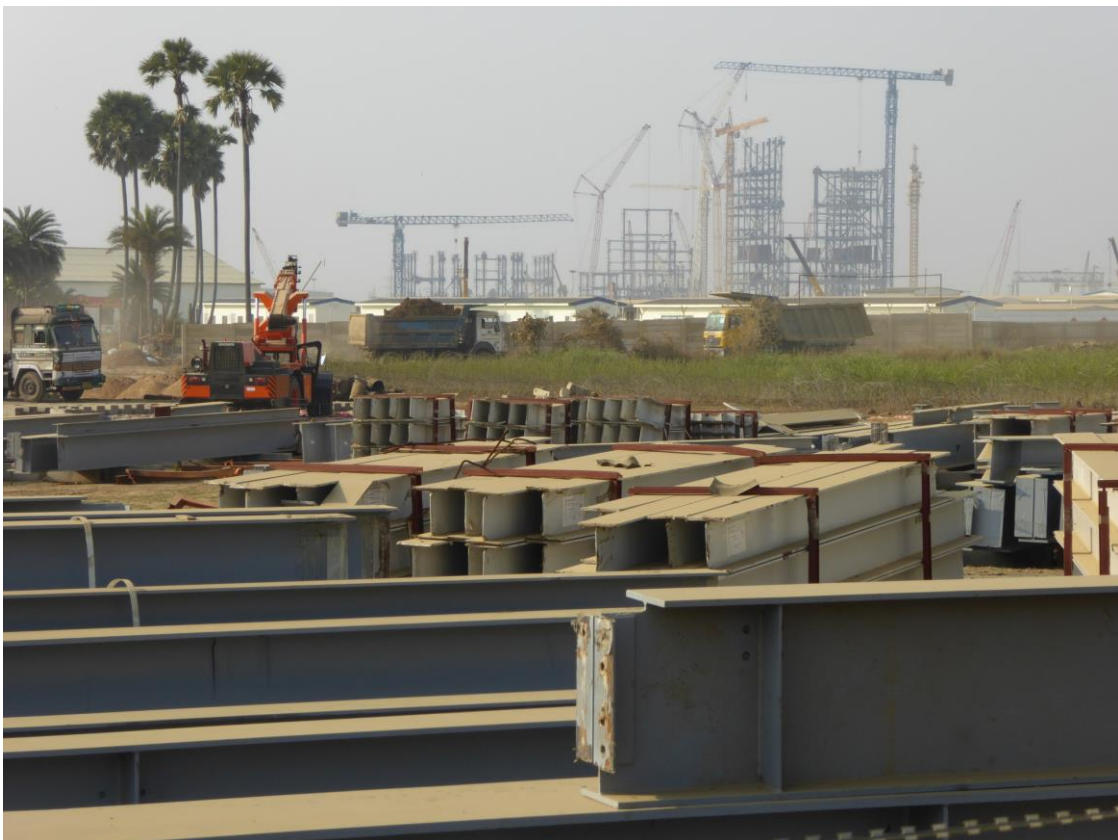
Construction of Adani's Godda power station proceeds on lands acquired from indigenous farmers near Godda. Photo by Geoff Law, February 2020
