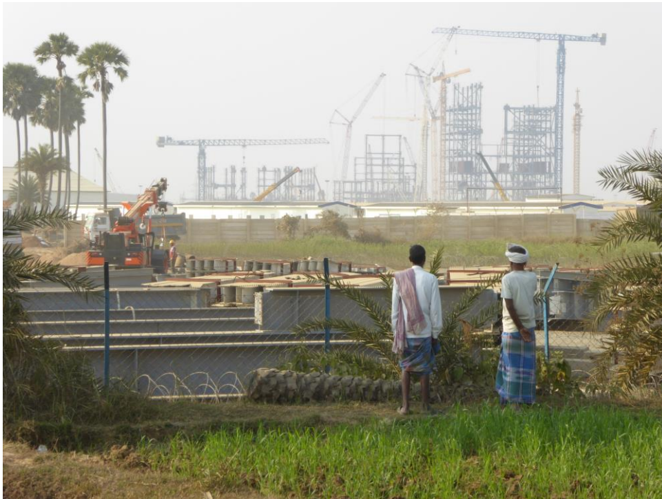
Construction of Adani's Godda power station proceeds on lands acquired from indigenous (Adivasi) farmers near Godda. Two Adivasi look on. Photo by Geoff Law, February 2020
