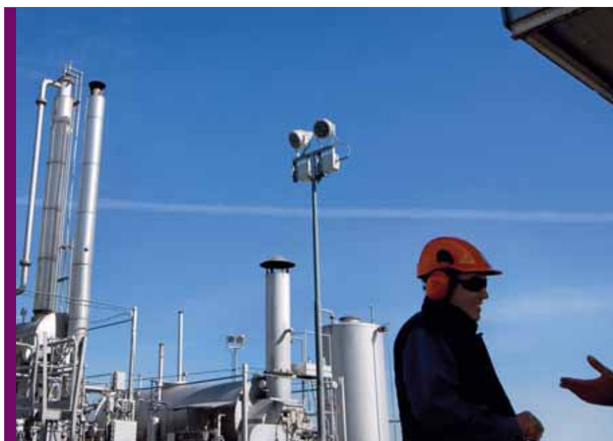
Edison has gas storage sites at Collalto and Cellino Attanasio (shown here). A third is being planned.
