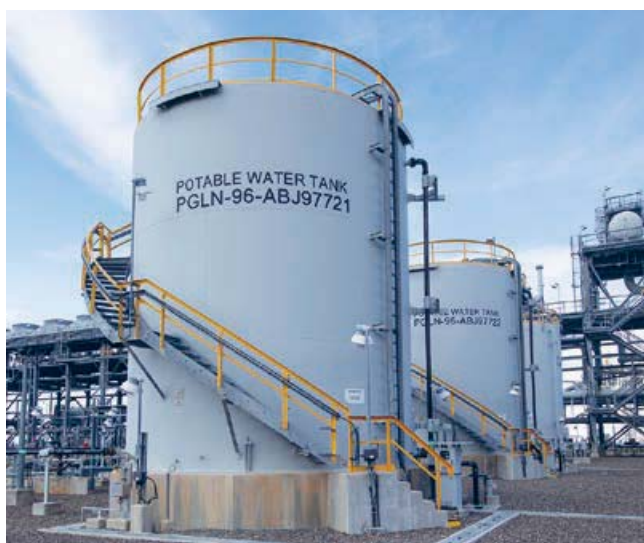
| One of two 260-cubic metre potable water tanks at the LNG Plant
