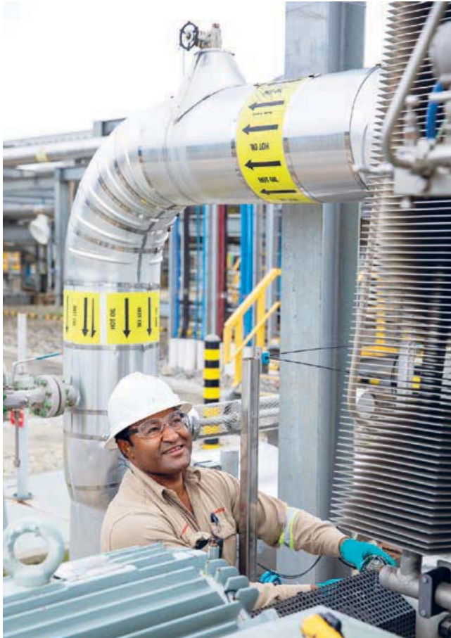
HGCP Mechanical Lead, Jackson Michael, conducts maintenance on the HGCP hot oil monoethylene glycol regeneration pump
