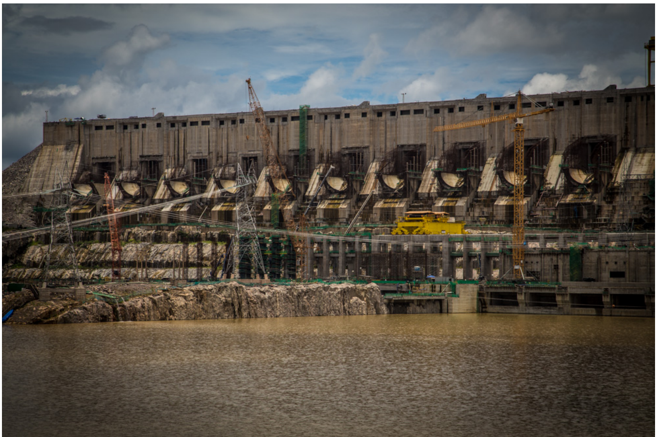
Belo Monte's main powerhouse, March 2016
