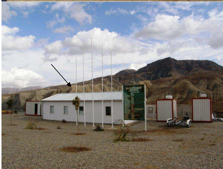
Photo 5: Ilisu construction site The first office barrack with the information sign post, located a short distance downstream of Ilisu village, so far is the only visible indication of the work starting on site. The arrow indicates the left bank dam crown abutment.
