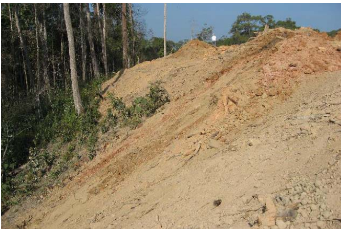
Spoil is still being bulldozed over the edges of the dam site road destroying living trees and threatening the Nam Theun below.
