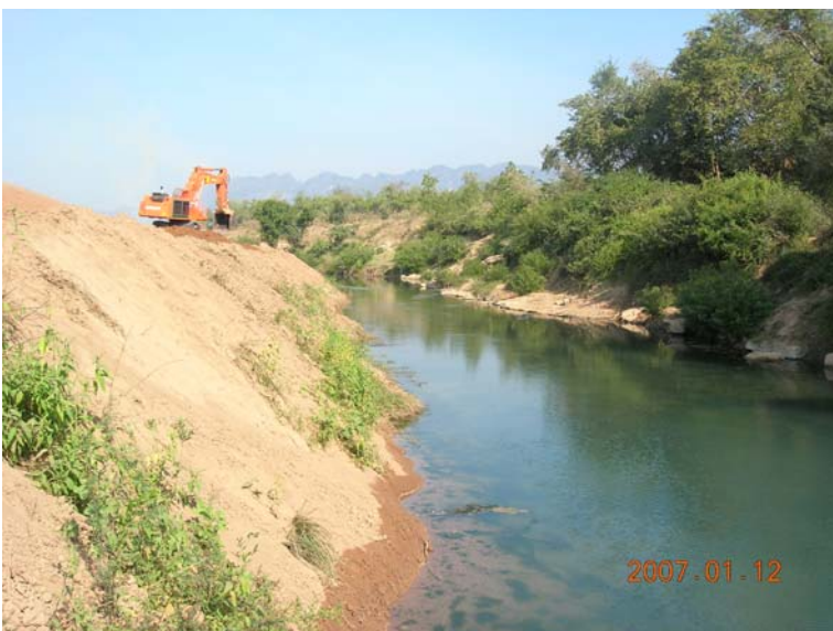
The Nam Phit being converted from a free-flowing river into a water channel.
