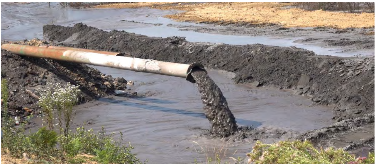
Image 4.4. Hydraulic transport of ash and slag from the Tuzla power plant to Jezero II ash disposal site
