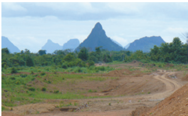
Land preparations in Fuang District for the resettlement of 6,000 people for the Nam Ngum 2 Dam.
