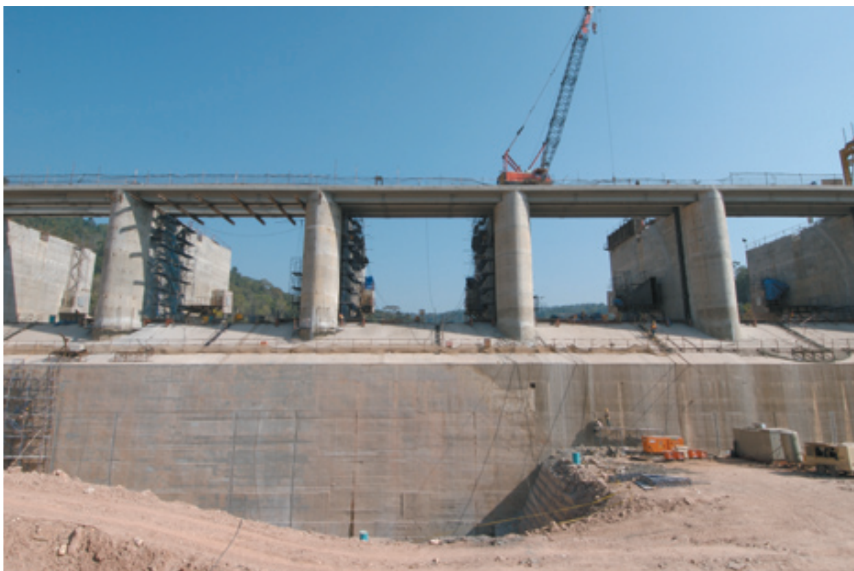
Sluice gates under construction at the Nam Theun 2 Dam. Photo: © Marcus Rhinelander
