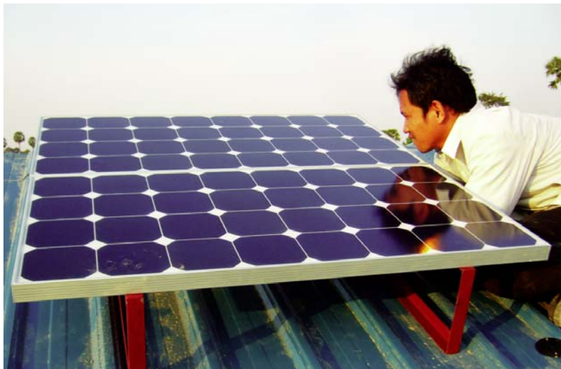
Installing a solar panel on the roof of a security guard post in Kampong Speu province to supply solar lighting in the evenings. Photo courtesy of Clean Energy Group.
