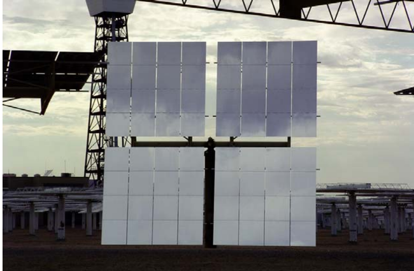
10 MW Solar Thermal Power Plant in California, USA. Photo courtesy of kjkolb.
