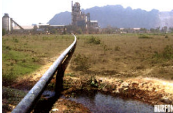
Kanbauk Myaing Kalay gas pipeline
