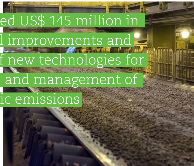
Pellet belt conveyor at the Pelletizing Plant of the Vargem Grande Complex, in Nova Lima (MG, Brazil) Photo: Marcelo Coelho
