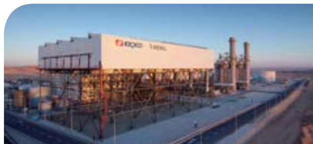
Power plant in Al-Qatrana, Jordan
