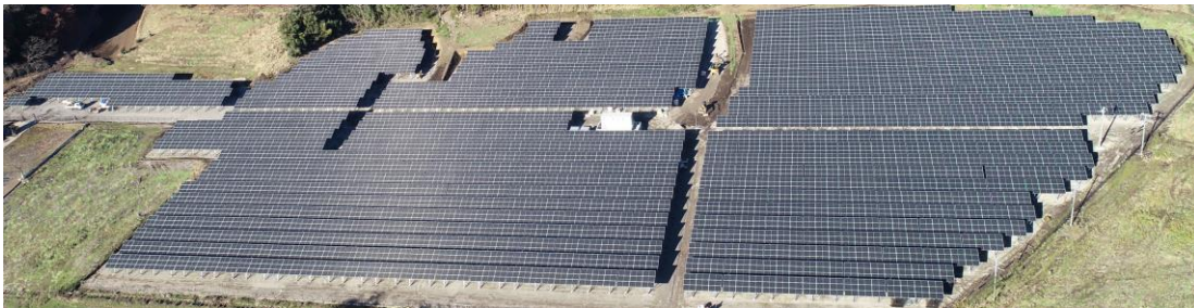
Figure 2-8 Offsite Corporate PPA (Ibaraki Prefecture)
