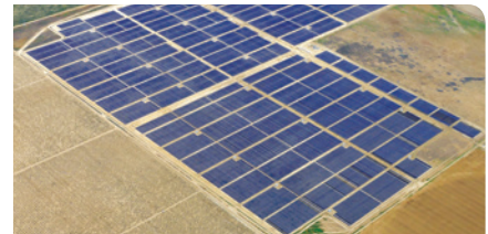
This Solar Flow-Through Fund 600 kw DC site, which is located in the Greater Toronto area, was serviced by Panasonic and PNC Canada. For the next 20 years, this project will produce green electricity for Ontario's electrical grid.
