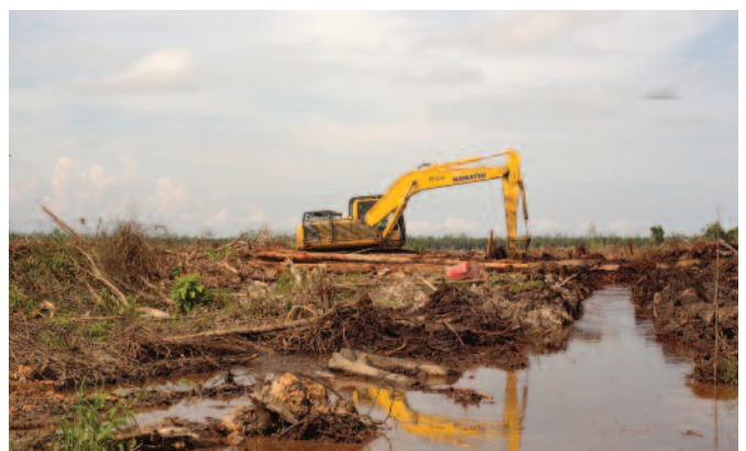
New land clearing, digging of drainage canal in Indonesia. © Jason Taylor / FoEI
